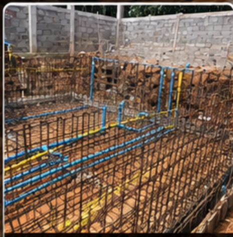
MAIN CIRCULATION PIPING
